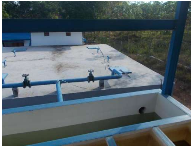
Gambar 3.33 Unit Reservoir IKK Sungai Pinang
