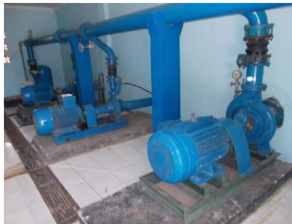
Gambar 3.31 Pompa distribusi PDAM INTAN BANJAR
