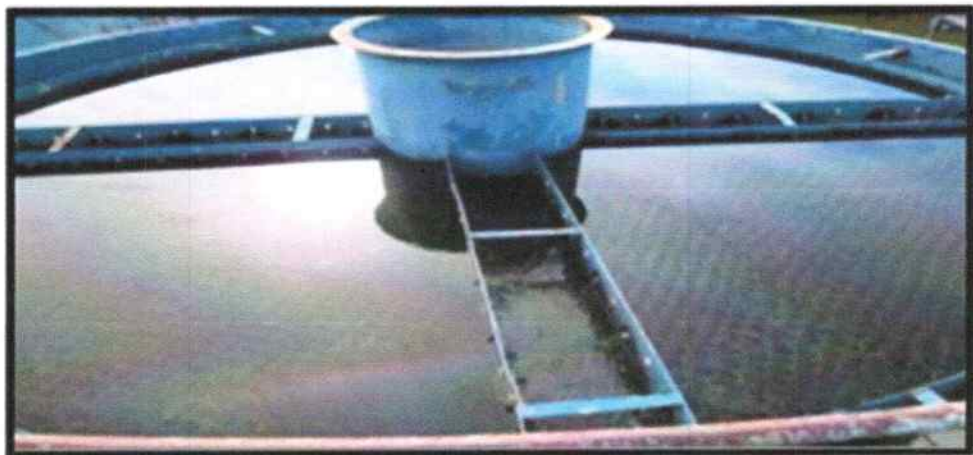
Gambar 3.16 Flokulator, Tube settler, Gutter
