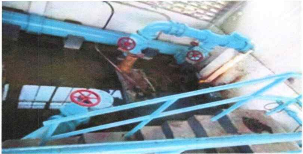
Gambar 3.19 Unit Pompa Backwash
